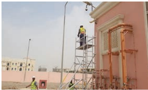
DEWA 132KV SUBSTATION
